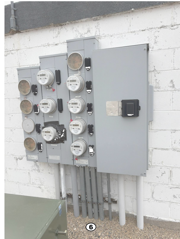
EXTERIOR NORTH WALL OF VAULT BLDG (UAC) (BID ALTERNATE 2 & 3) NOT TO SCALE
